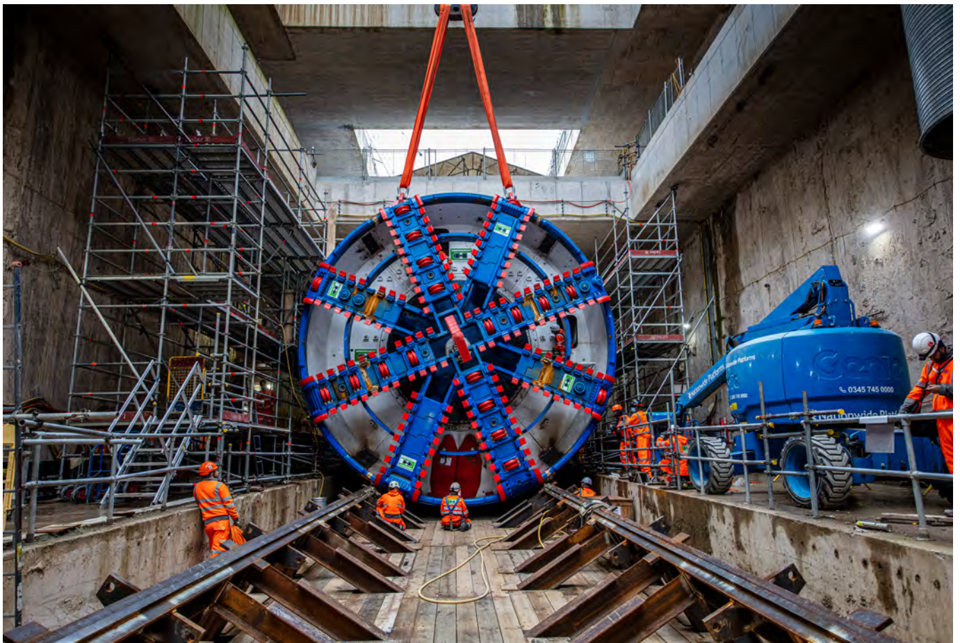
The cutterhead of the tunnel boring machine being lifted into the east box at Old Oak Common station
