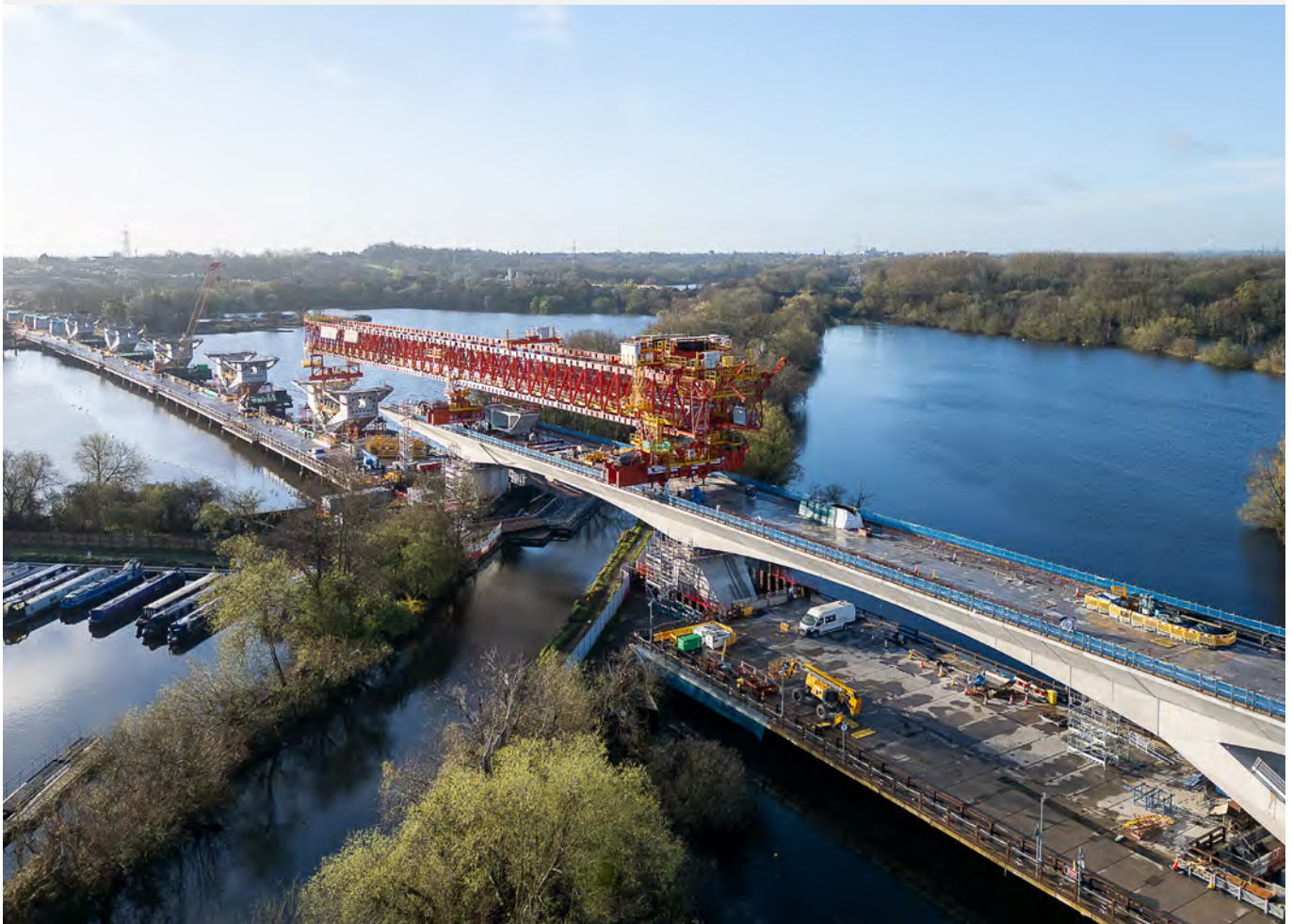
An aerial view of Colne Valley viaduct under construction. The launching girder lifts 140 tonne deck segments into place as the viaduct crosses the Grand Union Canal, which can only be conducted during periods of low wind speeds.
